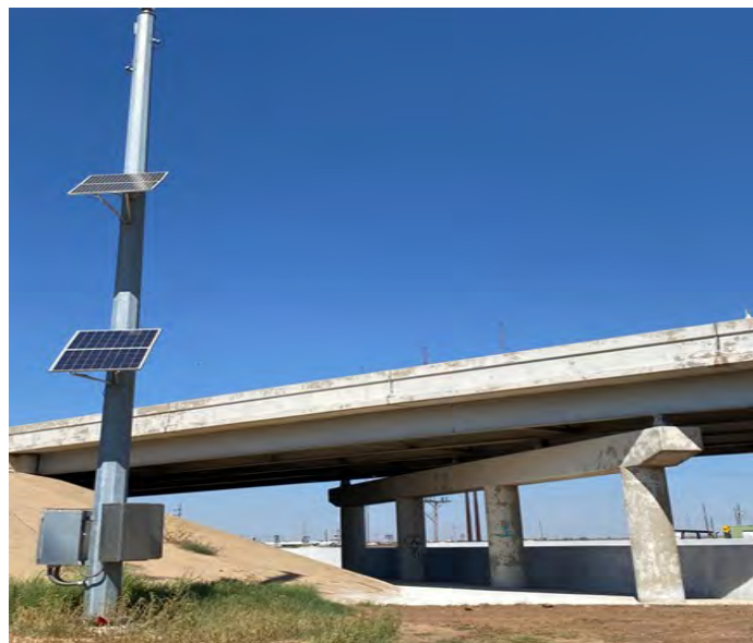
Pole with 2 solar panels and 2 battery cabinets.
