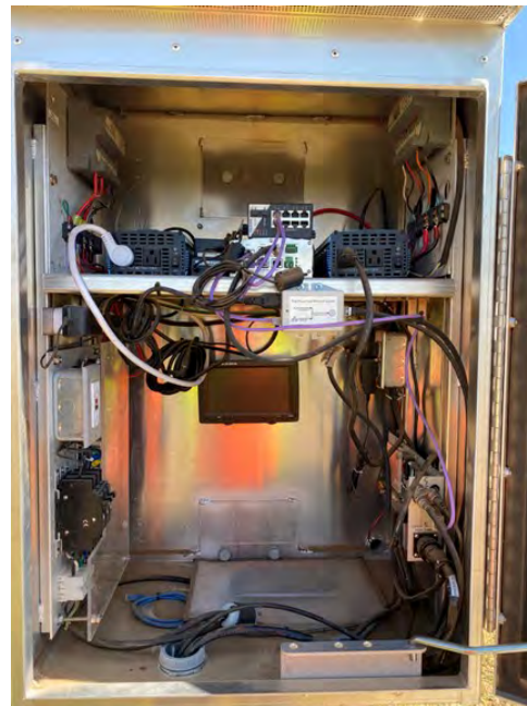
Inside solar CCTV cabinet. Shows standard TxDOT CCTV cabinet with two inverters to convert 12-volt DC power to 120-volt AC power for all components. Each solar system runs one inverter with specific equipment powered from each inverter to equally balance the electrical demand (load).
