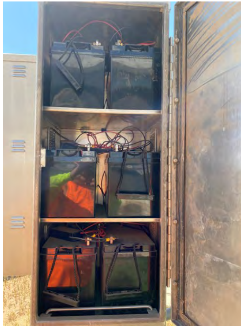
Six batteries are used per system and are wired in parallel for greater capacity.
